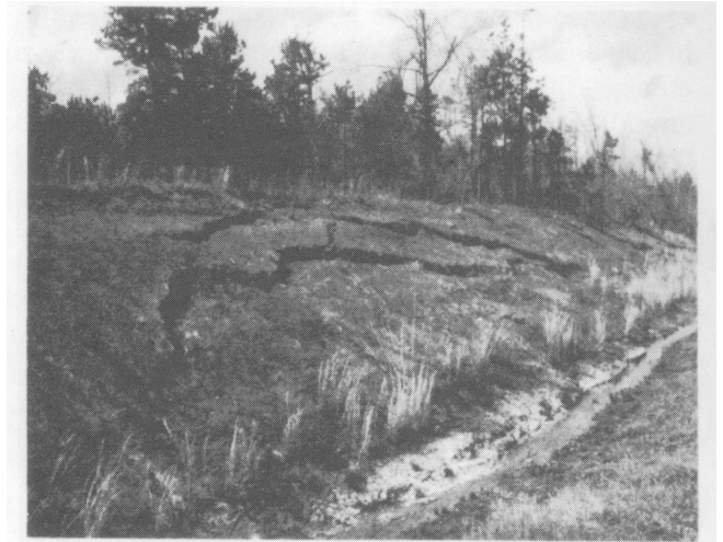
Figure 2-5. - Unstable Soil Conditions, as on this roadbank, should be avoided.
