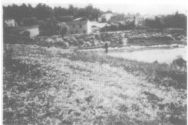
Figure 2-12. - This temporary sediment basin effectively trapped sediment from upstream erosion.
