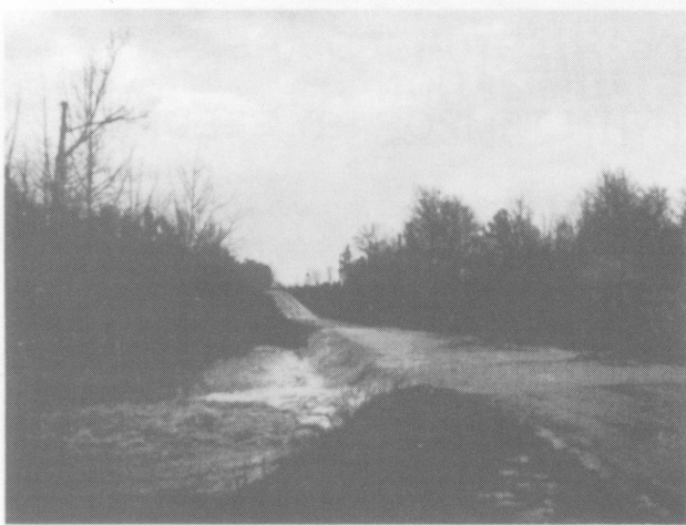
Figure 2-14. - An undersized culvert in this roadway has created an obstruction to floodwaters.
