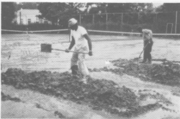
Figure 1-4. - Removing sediment from this tennis court was a costly and time consuming operation.
